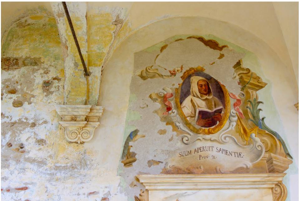
Fig. 8 – Painting on the top of “O” cell in the north arm. Decay phenomena show the different paint layers (white, yellow, green), the plaster cut surrounding the painting and traces of green paint close to the painting (photo by the authors, March 2019).
