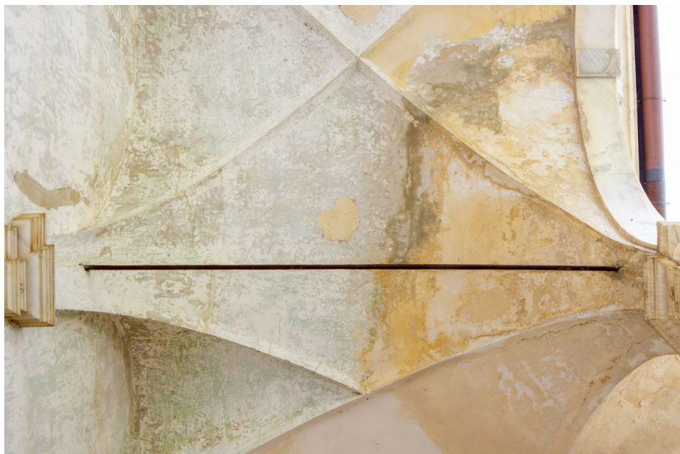
Fig. 3 – Vault intrados in the south arm. Green paint traces are appearing under two layers of different yellow paint (photo by the authors, March 2019).
