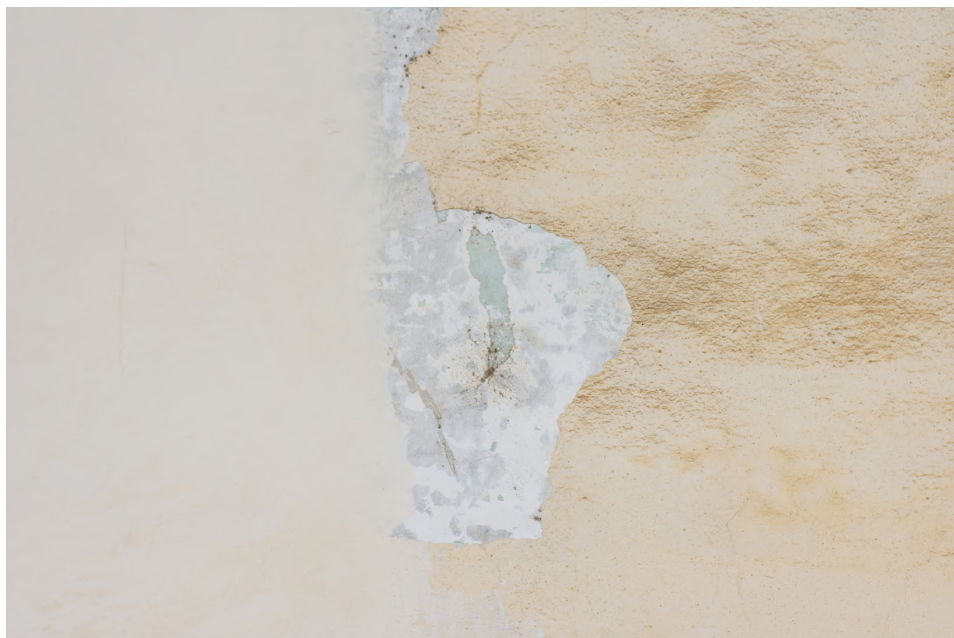
Fig. 5 – Two different plasters between the sixth and seventh spans of east arm. The colour, the thickness and the grain are clearly different (photo by the authors, October 2019).
