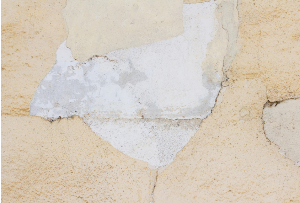
Fig. 9 – Horizontal plaster cut on the south arm and two different yellow paint layers (photo by the authors, October 2019).
